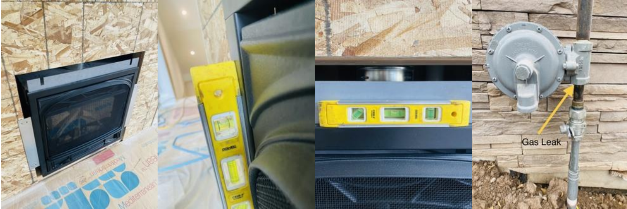
Unit set and leveled, location of gas leak outside.
